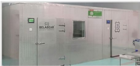
North American Candy Drying project
